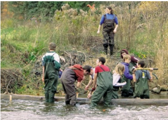
Young work crews installing cover structures at Camp Sidrabene on Bronte Creek, ON...
